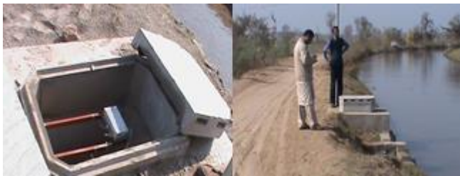
Fig. 1. Photographs of smart water meter installations in Bahawalnagar on distributary canals. The meter is mounted inside a concrete stilling well [2][8]
