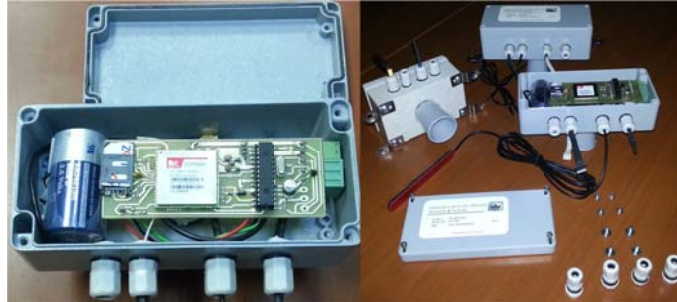
Figure 2(b): Photographs of the developed Smart Water Meter.
